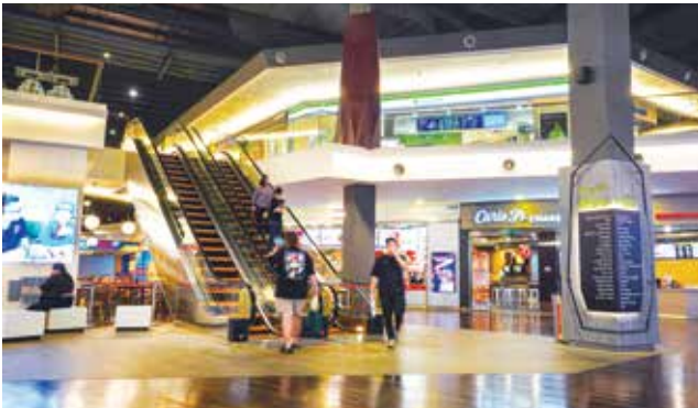
Replaced the North and South escalators connecting the Third Floor to the Third Floor Mezzanine at MVM
